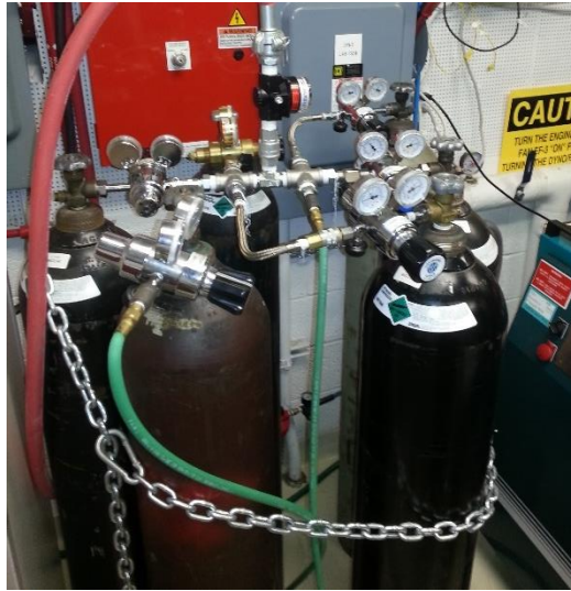
Figure 5.2: 6-cylinder N 2 and its manifold
